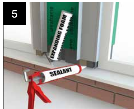
Weatherseal any joints/gaps under column and between windows/doors and columns. Use foam and/or appropriate sealant.
